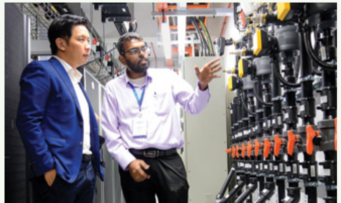
Singapore's Minister of State for Trade and Industry Mr Alvin Tan (left) touring the new Sustainable Tropical Data Centre Testbed. Credit: NUS.
