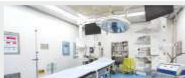
STATE OF THE ART OPERATION THEATERS 10 Ultra Modern Modular OTs with Modular Workstation, Laminar flow and HEPA Filters
